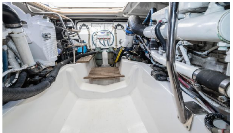
Engine room looking aft
